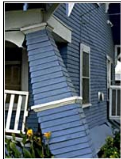
Figure 10 Earthquake Damaged Porch
