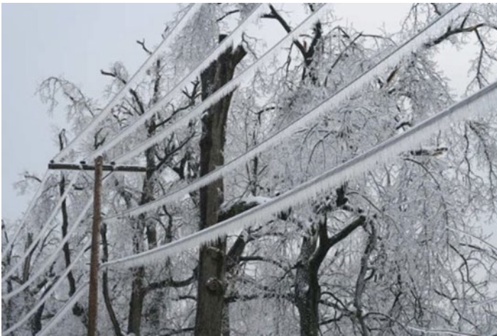
Figure 28 Ice Covered Power Lines
